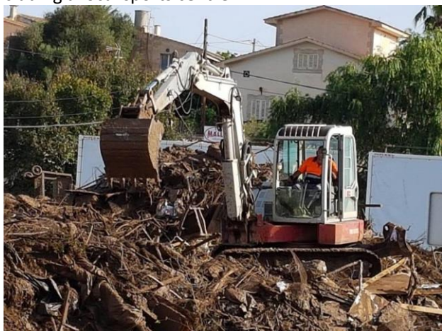
Figure 5. Clearing flood damage in Mallorca, Spain, October 2018 – Credit: 112 Illes Balears
